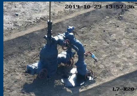
oil leakage identification
